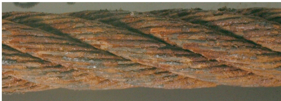
Figure H.3 — Surface of wire now greatly affected by oxidation — Rating: 60 % towards discard
