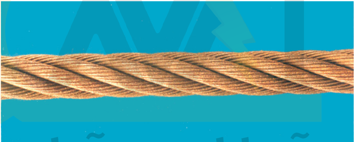
Figure B.11 — External corrosion
