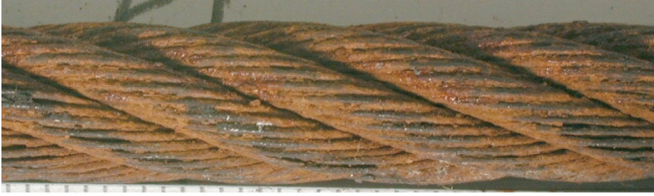
Figure H.4 — Surface heavily pitted and wires quite slack, gaps between wires — Discard immediately
