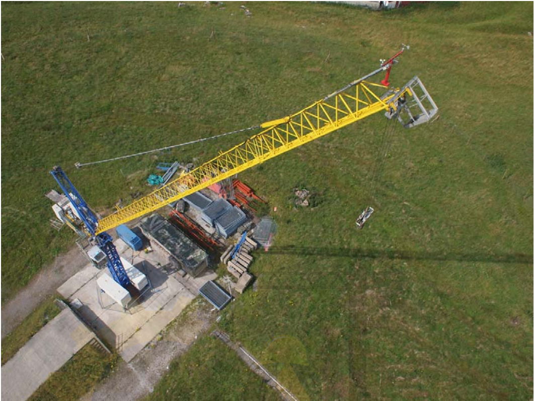
Figure 11a – General View of HSL Anemometer and Weather Vane fitted at the outer end of Jib Section 5
