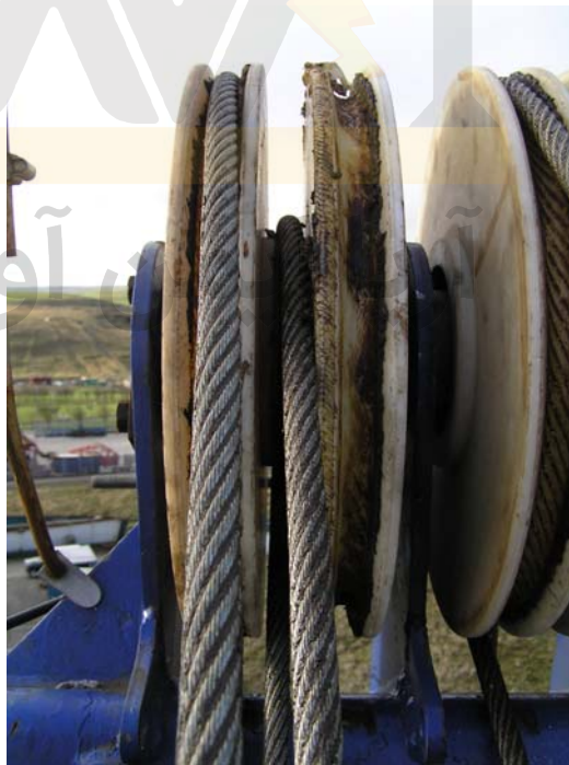
Figure 14b – Detail of the Luffing Rope out of the groove of the third ‘A’ Frame Pulley from the left (photograph is taken from the opposite side to that of Figure 11a)
