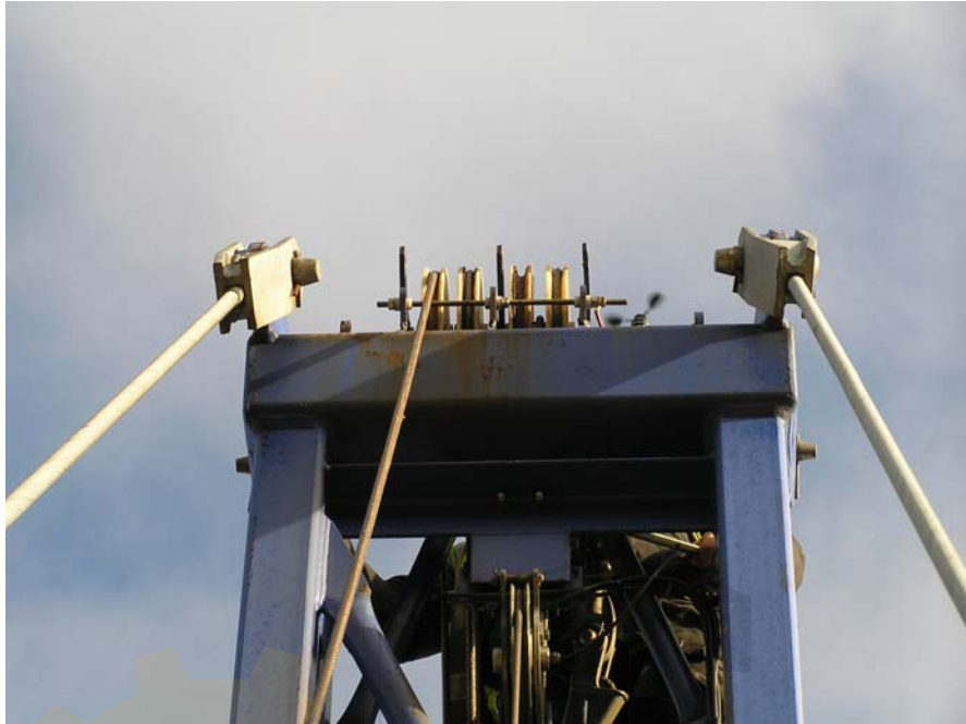
Figure 14a – General view of the Luffing Rope out of the groove of the third ‘A’ Frame Pulley from the left
