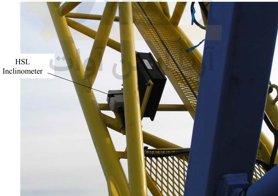
Figure 12b – HSL Inclinometer fitted close to the Crane Inclinometer
