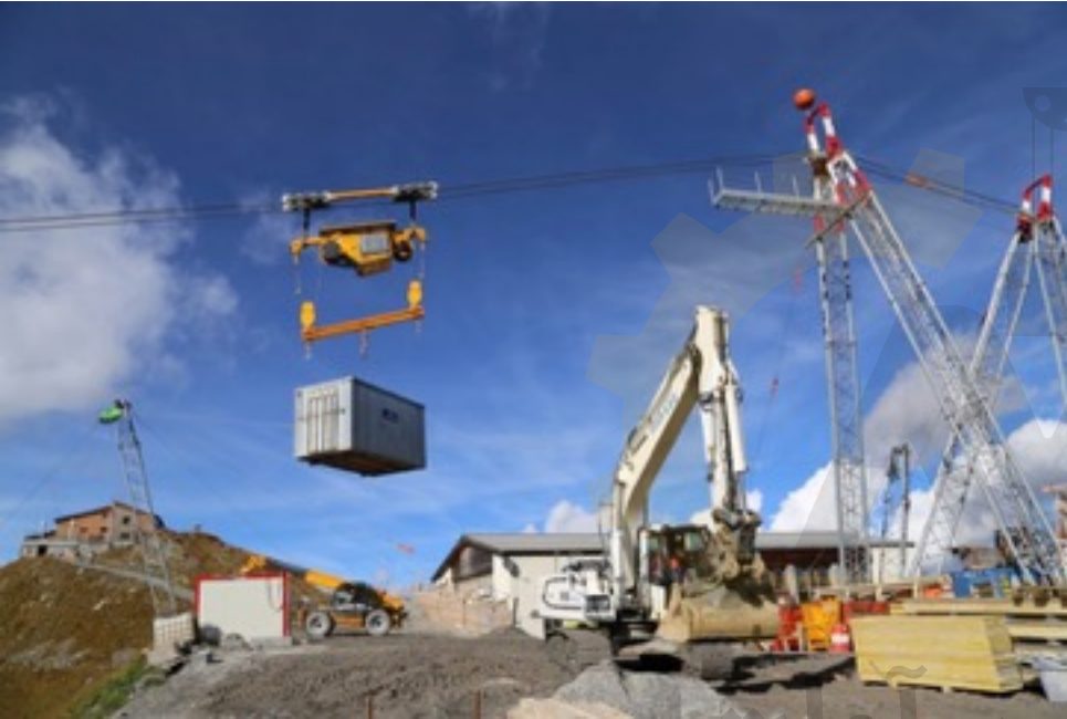
ASME B30.19 Cableway crane
